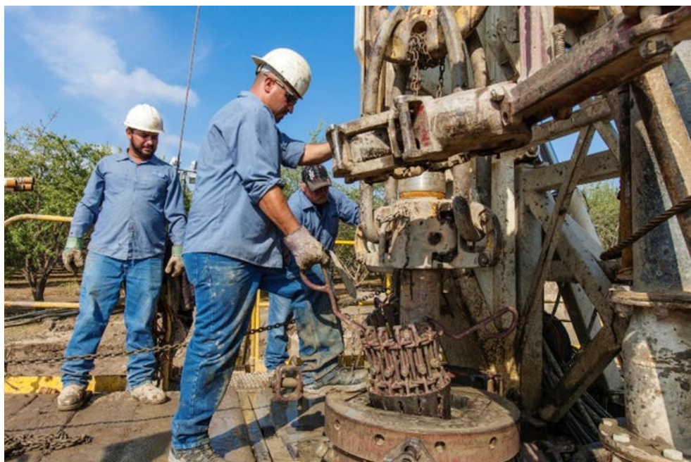
A new water well is drilled in an almond orchard in Tulare County in November 2014. During California’s severe drought, a record number of well-drilling permits were granted as farmers and others struggled to keep up with shrinking groundwater levels. Citizens of the Planet/Education Images/UIG via Getty Images
